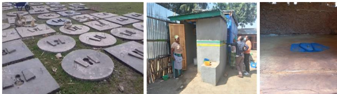
Figure 1: Slab manufacturing (left), construction of improved latrines (middle), and plastic slabs (right). Photo credit: Amref, BBBC and Plan international sub-programme offices
