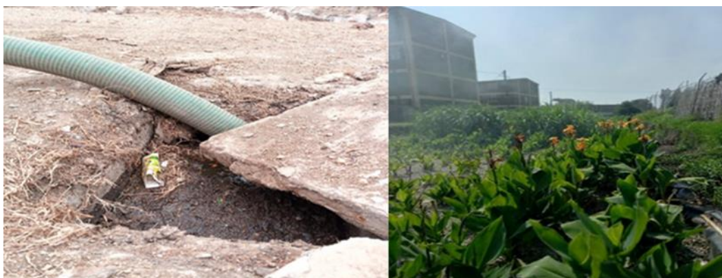
Figure 4: Septic tank (left) before and wetlands constructed (right) for sewage treatment in Shashamane. Photo credit: BBBC
